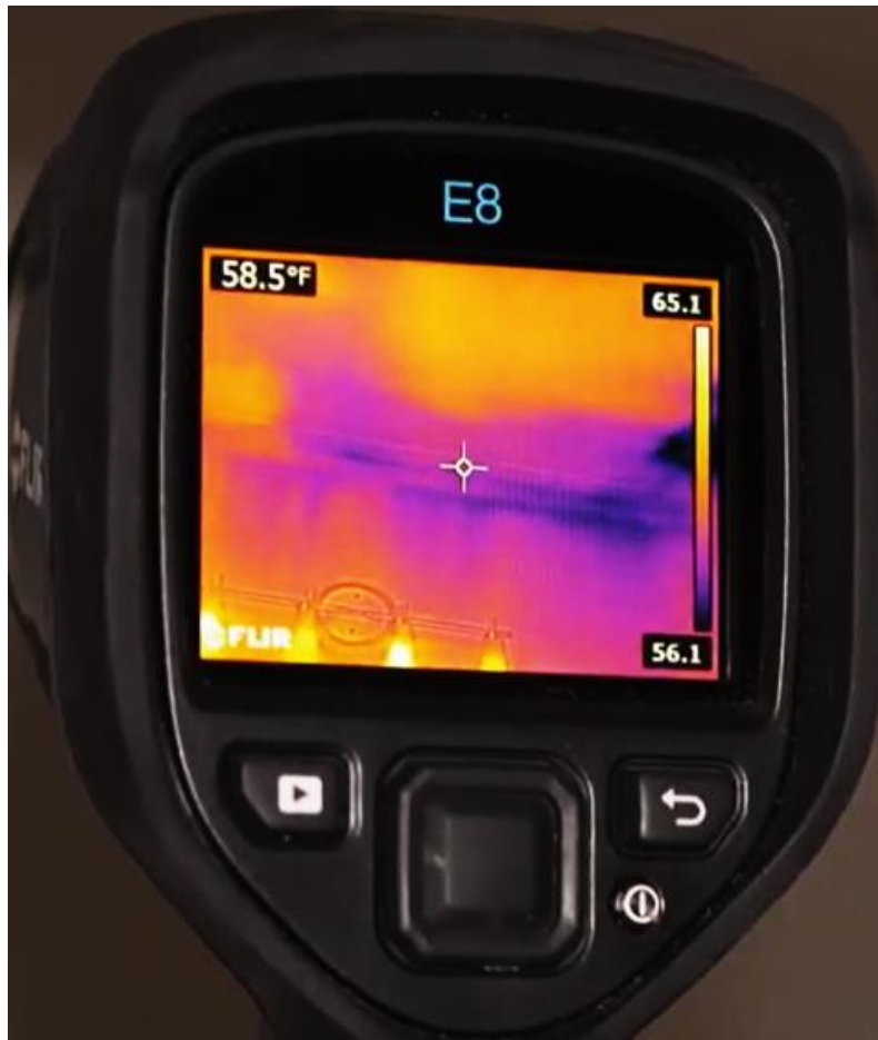
Cold air from an attic being drawn into a wall assembly by a blower door cooling down the wall near the top plate.
